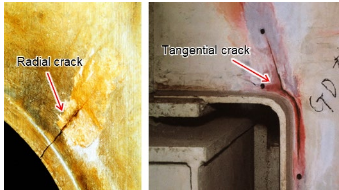
Figure 1-12 Fatigue cracking at cross-sectional changes [46]
