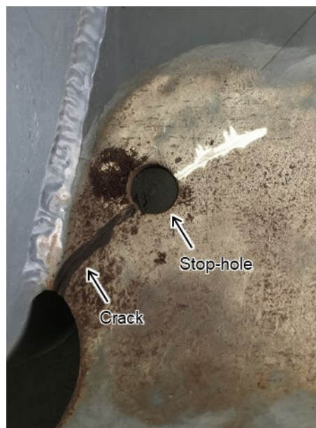
Figure 1-22 Stop-hole on a bridge diaphragm [68]
