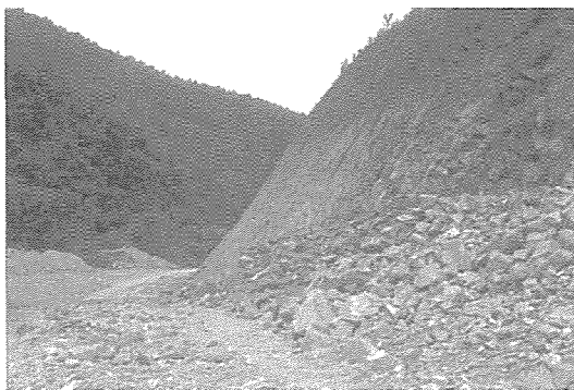
Photo 3.2. A new steep slope on the right side of Highway No.12
