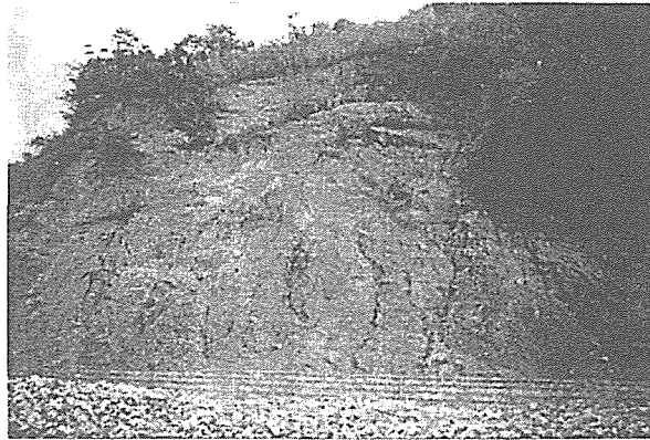
Foto1.1. Landslide in Huoi Leng Commune (350m of length, 150m of high with many terras )
