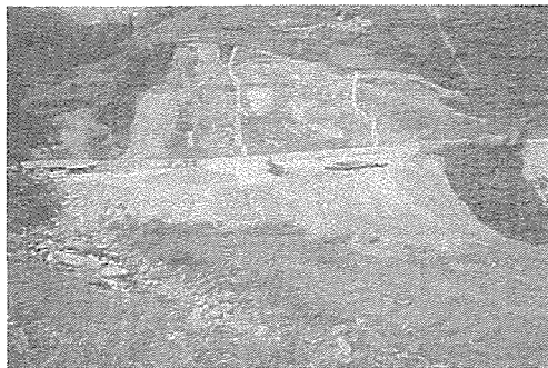
Pic. No1. The typical landslide point at Móng Sến II bridge, Sa Pa district, Lào Cai province occurred several times in recent years and caused large material damages and human losses (taken by Đào Văn Thịnh, 2002)
