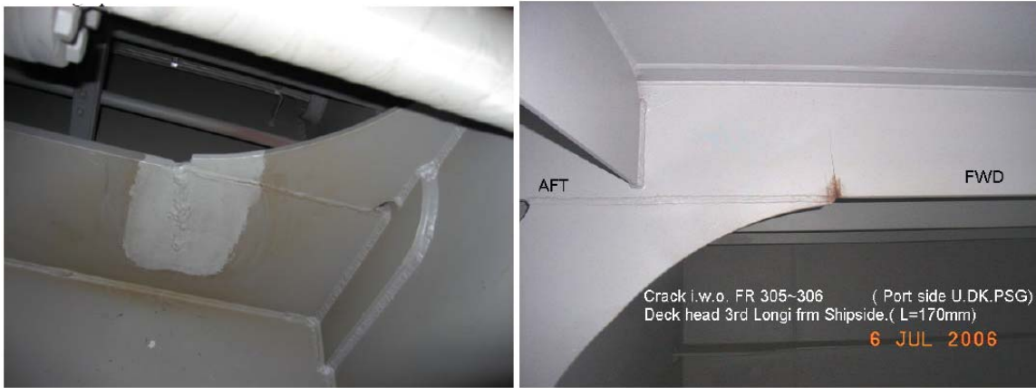
(a) a crack on upper inner side longitudinal (b) a crack in deck longitudinal
