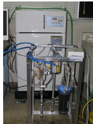
(b) Power supply and chiller
