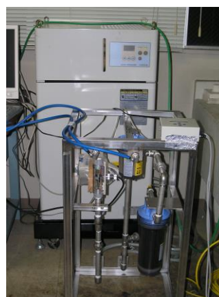
(b) Power supply and chiller
