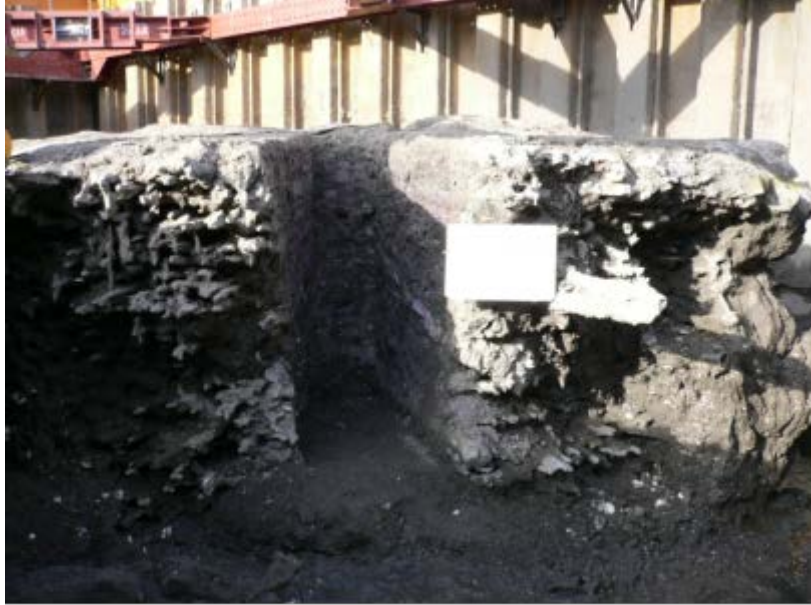
Fig. 4.19 Type 1 : JETCRETE column by the nozzle with flow conditioner with stepped rifting
