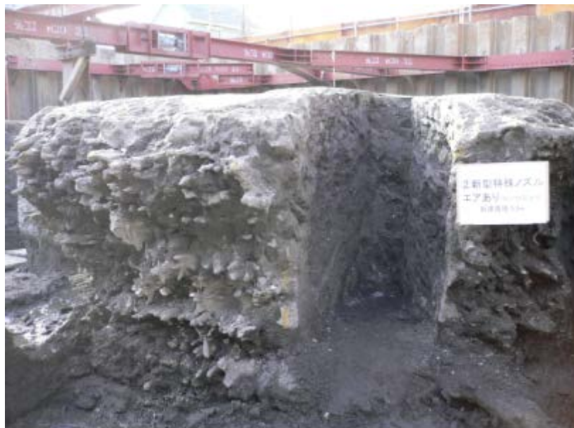
Fig. 4.18 Type 2 : JETCRETE column by the nozzle with flow conditioner with spiral rifting
