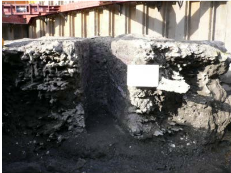
Fig. 4.17 Type 1 : JETCRETE column by the nozzle with flow conditioner with stepped rifting
