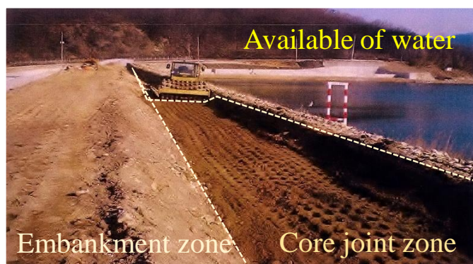
Figure 1.9 Heightening work for core heightening by inclined type (Site: Gyeryong reservoir, Gongju-si, Chungchungnamdo, South Korea, 2010)
