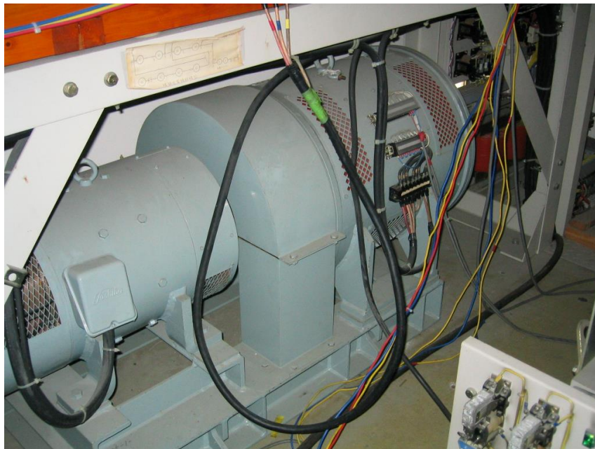
Fig. 3.25 Photo of synchronous generator moved by a dc motor.
