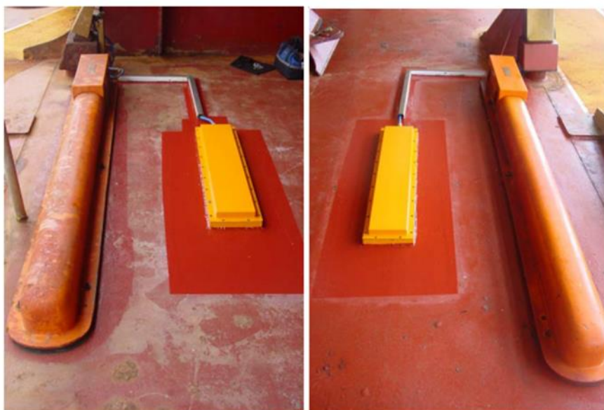
Fig.B.2 Life Time Sensor attached to upper deck of a FPSO.
