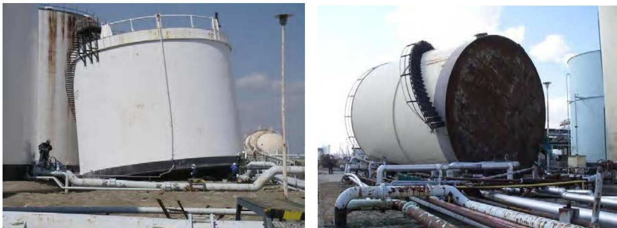
Fig. 1.2 Movement and tumbleness of large tanks (Fire Defense Research Centre, 2011)
