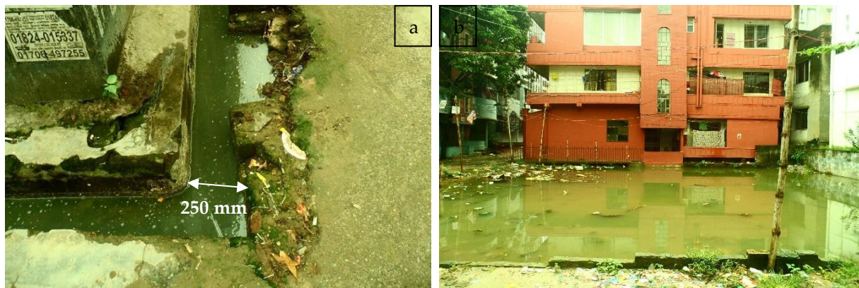
Figure 5. 4 a) Narrow drainage infrastructure and b) Inundation due to heavy rainfall and drainage congestion
