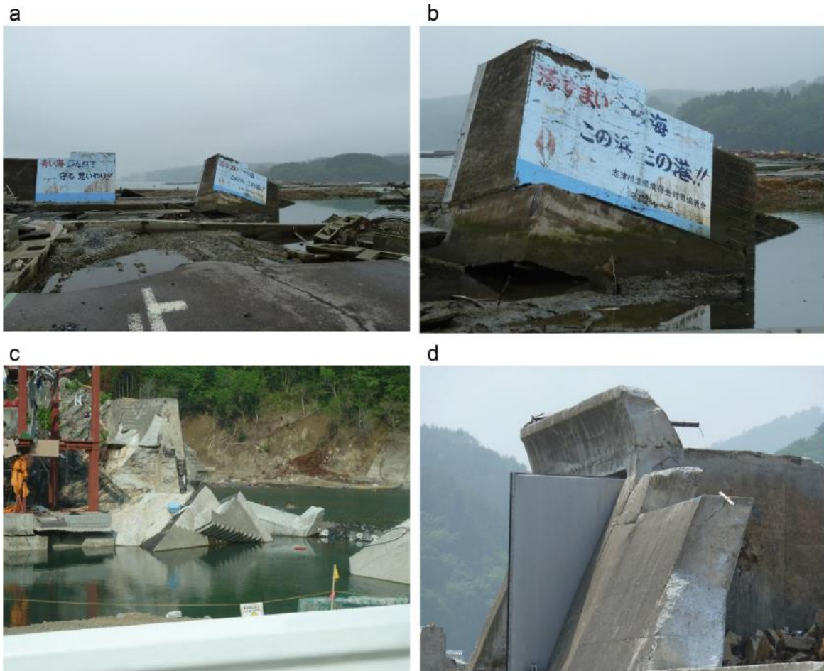
Figure 1.7. Seawall damage observed during the 2011 tsunami disaster: (a) damage to seawall and quay at Minamisanriku; (b) close-up of sea wall block at Minamisanriku showing no inter linkages; (c) recovery work on the seawall at MiyakoBay; and (d) remaining seawall buttress at Tarō.
