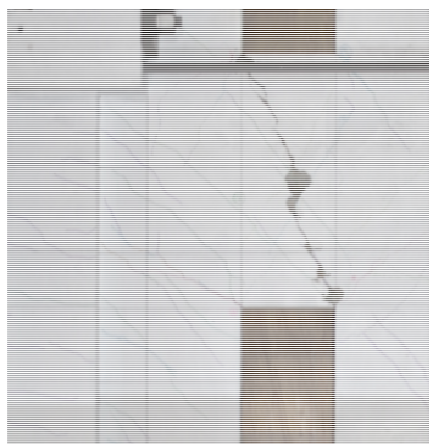
(g) Failure of the 3 rd floor beam ( R=+0.5\%rad )
