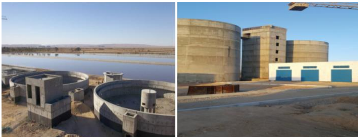
Figure 4- 3: Gafsa WWTP after rehabilitation and anaerobic digesters installation [126]
