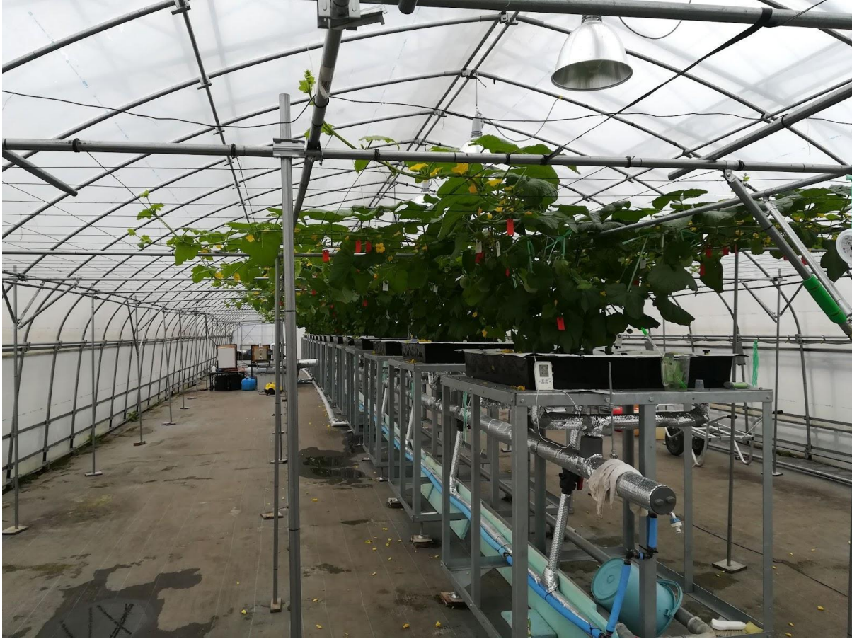
Figure 5: The melon greenhouse at Farm S, with a pipe carrying heated water using the excess heat of the biogas generator (photo by author).
